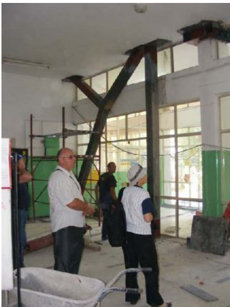
Internal bracing in the Electrotechnical school with dumper in right down corner
